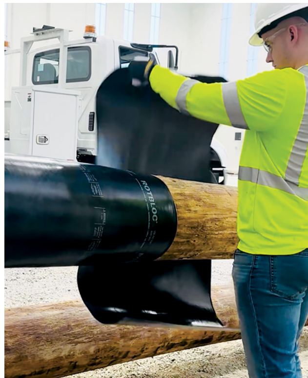
PHOTO: by Jessica Carhart of a ROTBLOC UTL on-site install by ALAMON, INC. who services electrical grids and utility poles nationwide.
